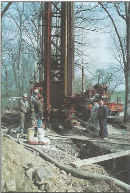
MCMUA Chief Engineer John Scarmozza, Water Superintendent Randy Stalter and Construction Inspector Frank Del Negro observe well-drilling operations at the new wellfield site in the Rockaway River basin. The MCMUA continues to explore groundwater resources to provide additional water supplies to Morris County municipalities. (Photo by Geoff Knapp)
