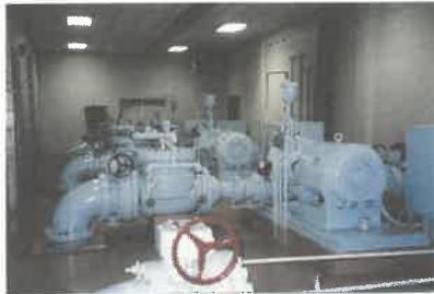
The well-maintained pump room at Markewicz Pump Station contains high-capacity pumps that deliver water to MCMUA customers.
