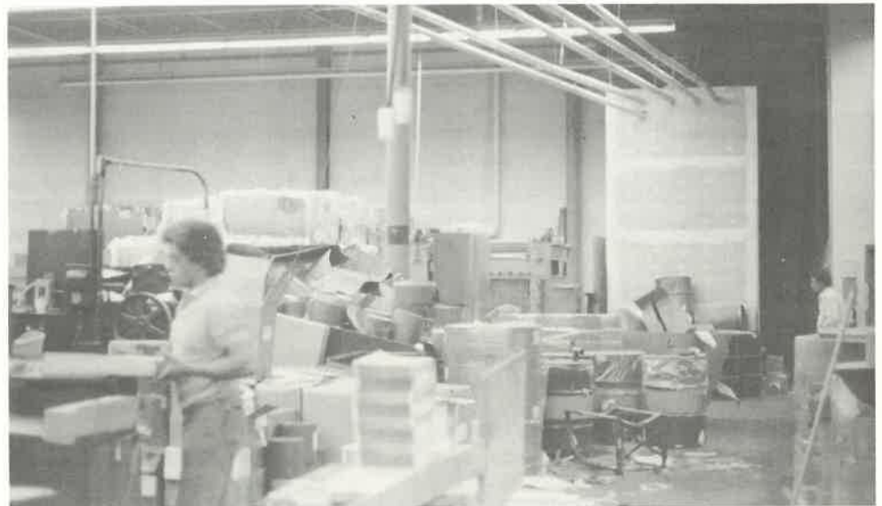
Paper is vacuumed into pipes and blown into a holding room (right rear), and then baled for shipping (left rear).
